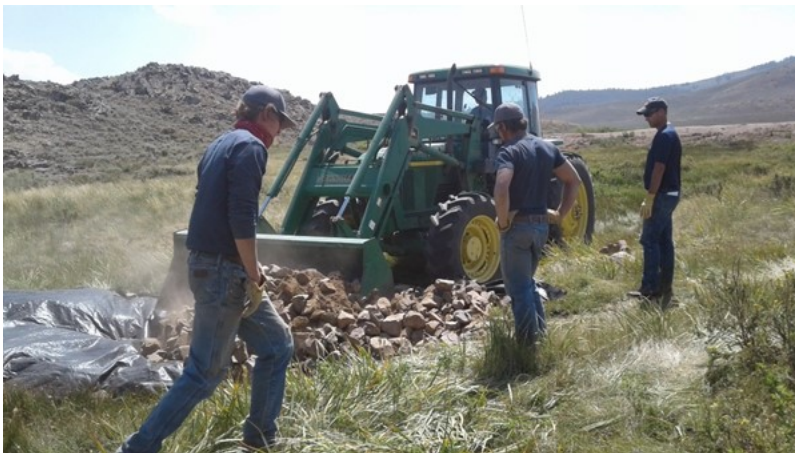
BLM Colorado and Colorado Parks and Wildlife construct a low water crossing used to maintain the water table in the meadow.
